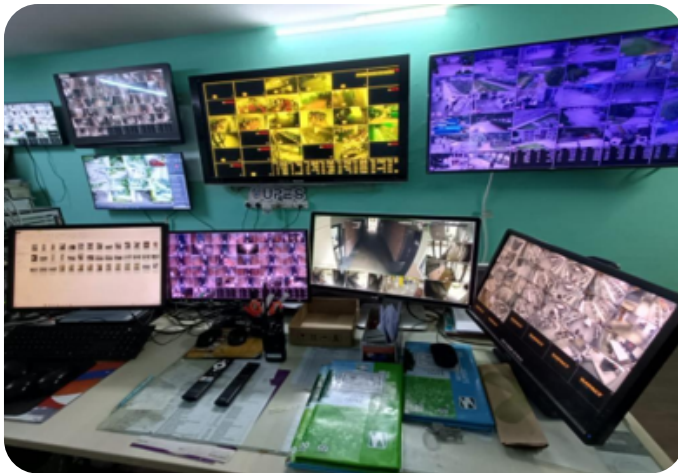
Central CCTV monitoring room
